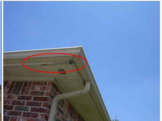
⌋ Fascia/trim boards are slightly water damaged at front right corner of dwelling.
