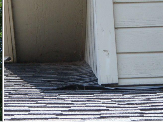
These Shingles at the right side of house need to be sealed so as not to have water or vermin intrusion.
