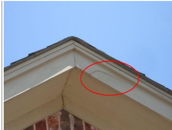
⌋ The fascia board at front is cracked.
