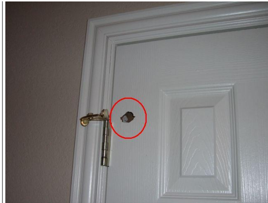
⌋ Wood damage at closet door in upstairs bedroom.
