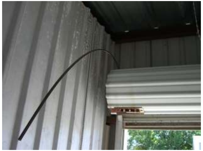
Unit 104 needs weather strip re-installed.
